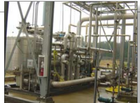
Skid mounted, 2,400 CFM, solvent recovery system at chemical manufacturing facility
