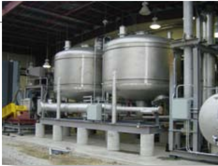
Skid mounted, 6,400 CFM, solvent recovery system at fiber manufacturing facility
