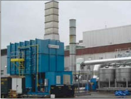
Oxidizer and skid-mounted carbon adsorption system controlling emissions from coating operation
