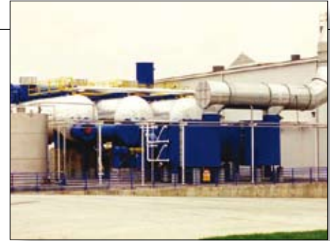
Large, 90,000 CFM, turnkey, solvent recovery system at adhesive tape manufacturing facility
