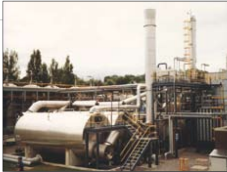
Solvent recovery system (carbon adsorption system and distillation system) at pharmaceutical firm
