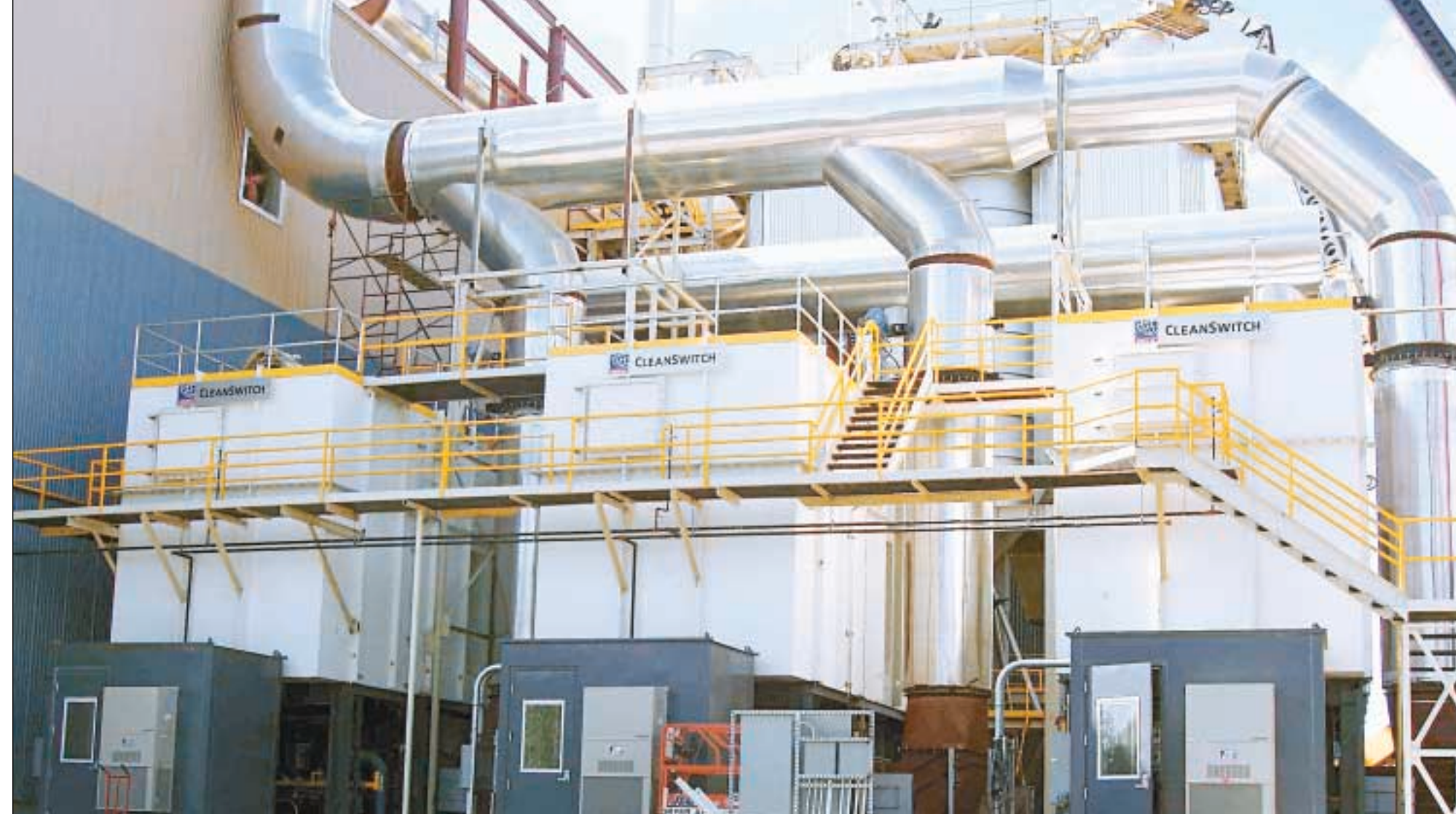
These three CleanSwitch RTO modules from MEGTEC Systems each have a rated capacity of 55,000 acfm, a thermal efficiency up to 95% and MACT-compliant emission rates. They handle the process emissions from the two OSB dryers used at the Norbord mill in Bemidji. Each dryer has a dedicated electrified filter bed (EFB) system to control particulate emissions.
